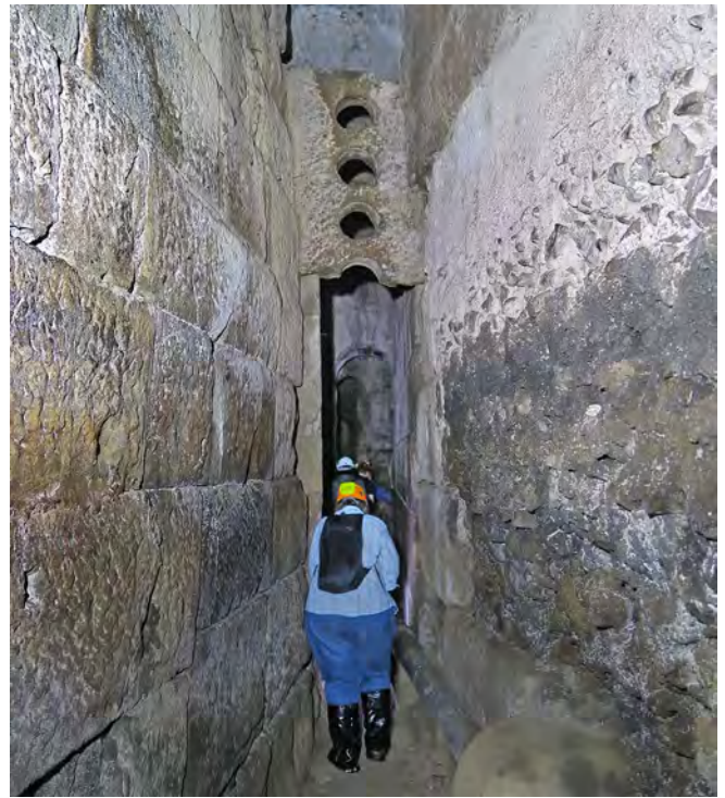
First entrance chamber of the Nemi drain, formed of cut tuff blocks. Today partially collapsed. Ahead is the upper surviving section of one of two stone debris barriers to stop branches and similar entering; circular holes allowed the flow of water. Maintenance and clearance of the chamber was via access shafts
